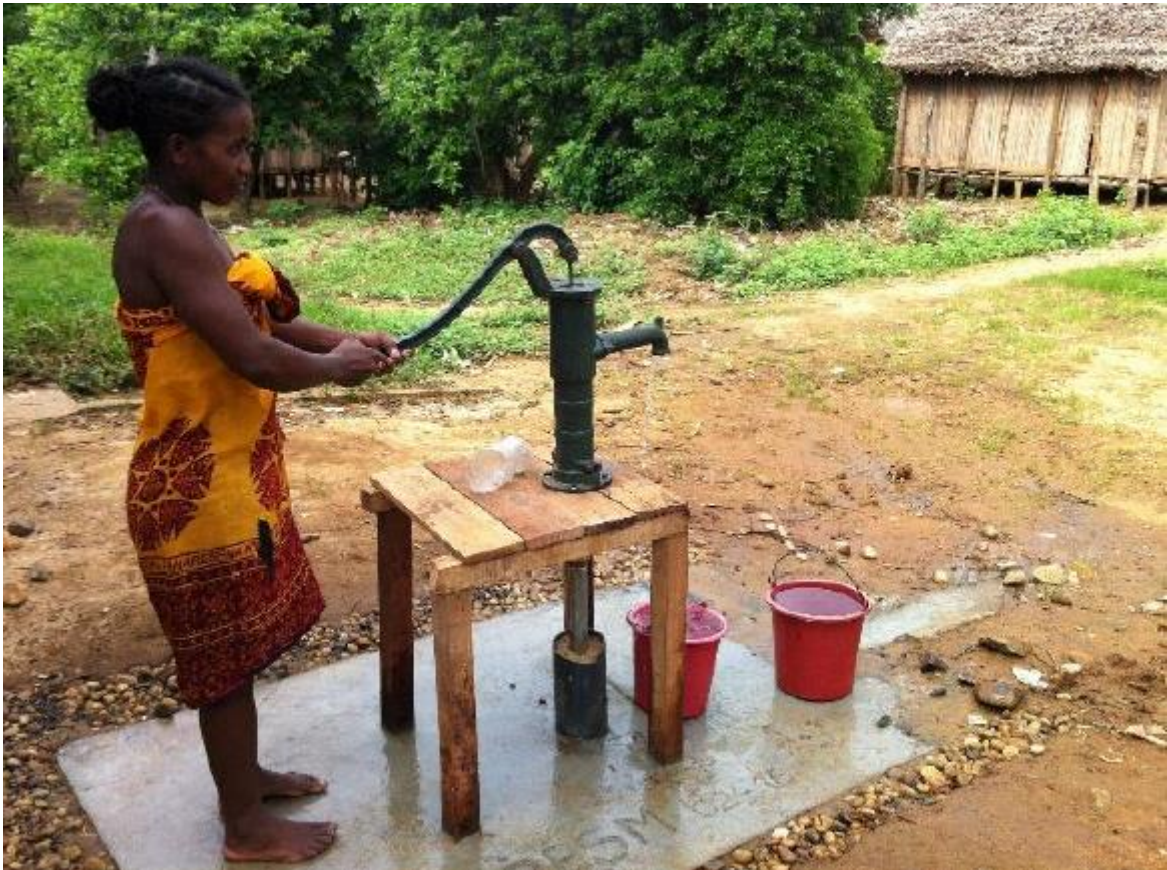
(Figure 1.2: MWP hand-pump in Tsivangina locality. Source: The MWP, 2016)
