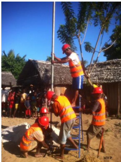
The team introducing the filter and the galvanised pipe into the borehole
