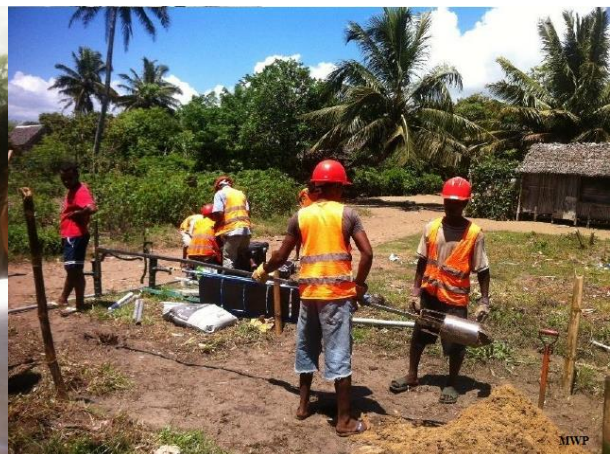
The auger is emptied and put back in the soil for continuing the drilling
